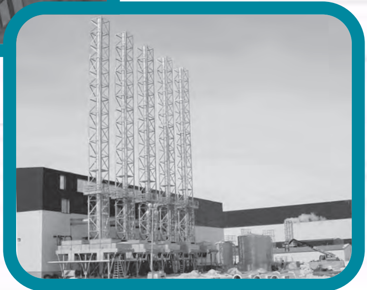
Generator & Fume Exhaust
