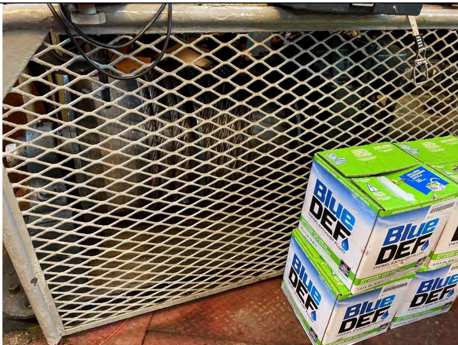
Description: Winch assembly; 10 gallons diesel exhaust fluid bottom right corner; blueprint ref. W
