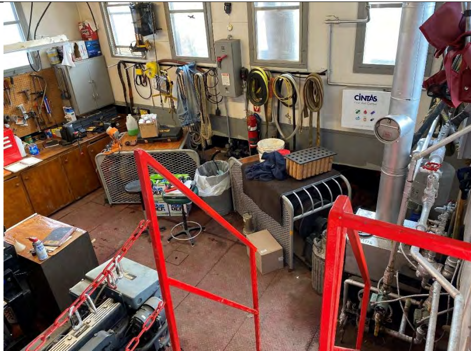
Description: Engine room
