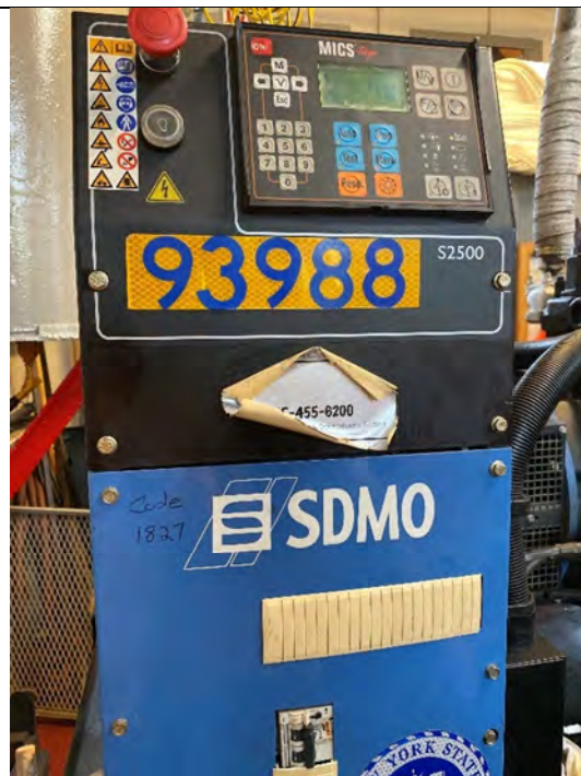
Description: SDMO generator and control panel; blueprint ref. L
