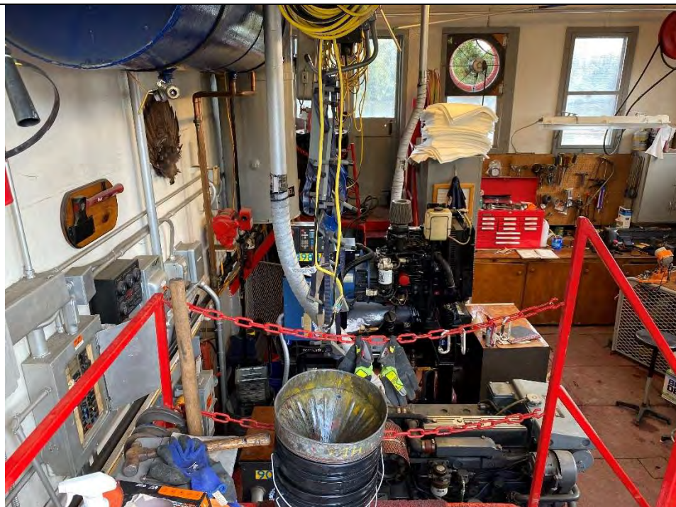
Description: Engine room
